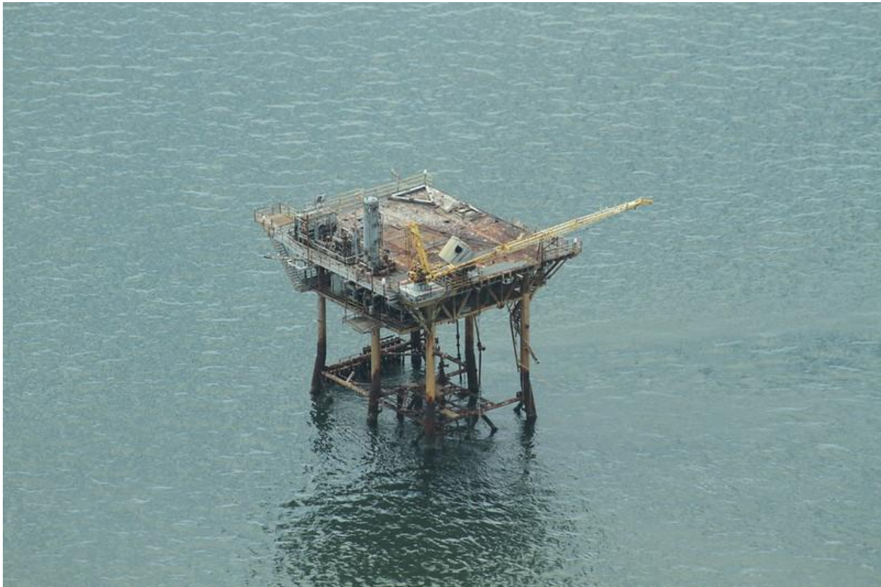
Figure 1. Deteriorating platform in Grand Isle Block 41. Credit: Healthy Gulf, March 2024.
