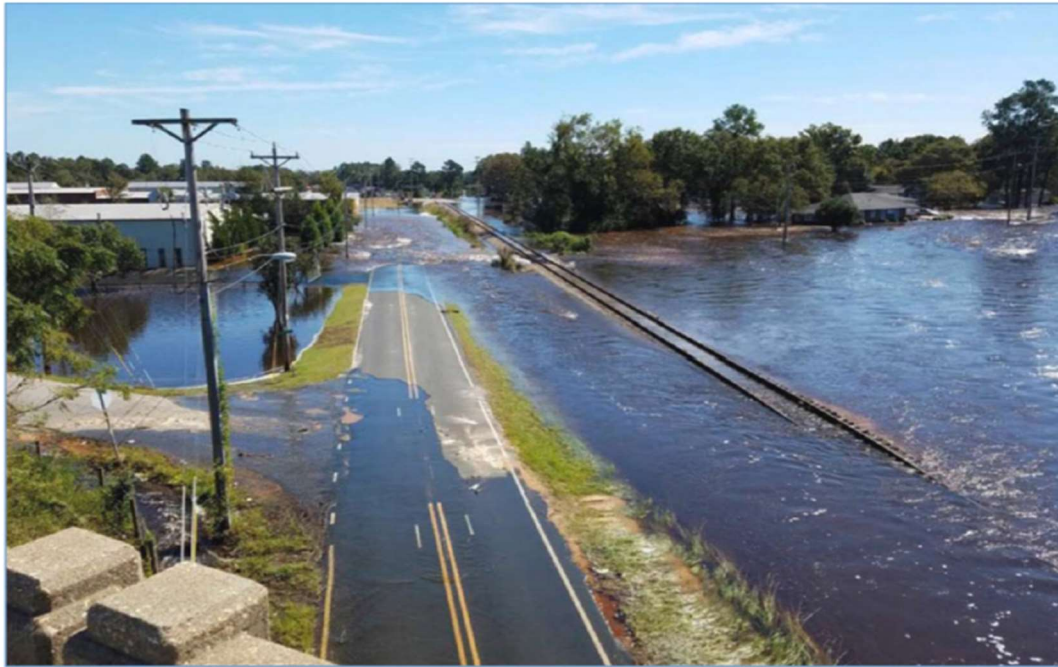
Figure 7: Water flows south from VFW Road Underpass Washing Out Railroad and Overtopping VFW Road
