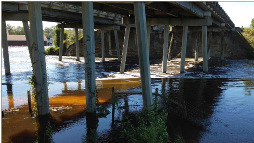
Figure 8: I-95 Abutments Eroded on SW Side of Underpass. Railroad not Apparent
