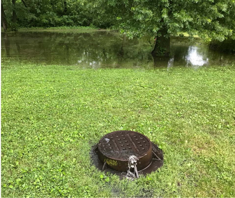
Figure 9: Manhole discharging sewage on June 30, 2020, near 466 North 73 rd St. in Centreville, Illinois.
