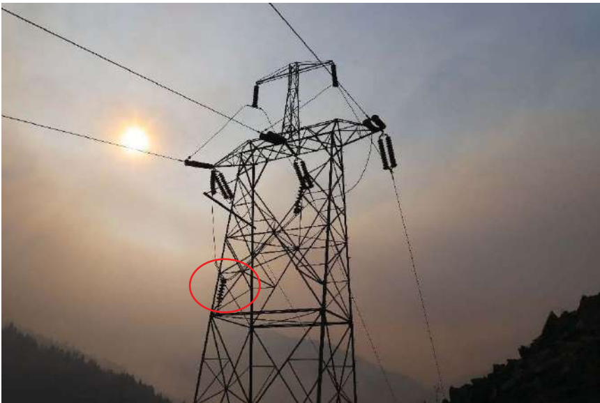
Figure 3. At the Incident Tower, an insulator detached from the hanger plate and hung upside down. Photo provided by PG&E. 79
