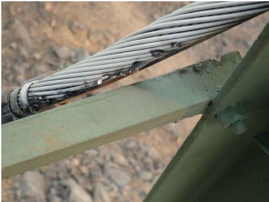
Figure 5. Flash marks on the transposition jumper and steel member on the Incident Tower. Photo provided by PG&E. 81
