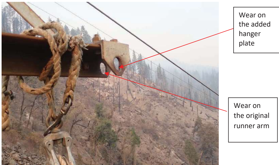
Figure 7. The right runner arm and the added hanger plate from the Incident Tower prior to removal from the tower for evidence. Photo provided by PG&E. 83
